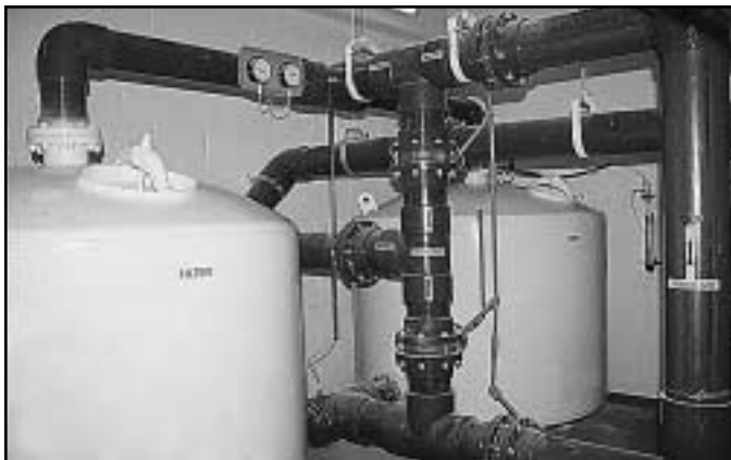
Sand filter system.
