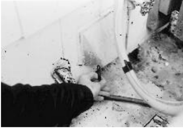
Figure 3.10. Rat entry point
