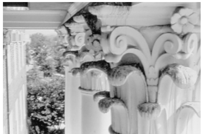
Figure 18.4. Defacement of building from pigeon droppings.
