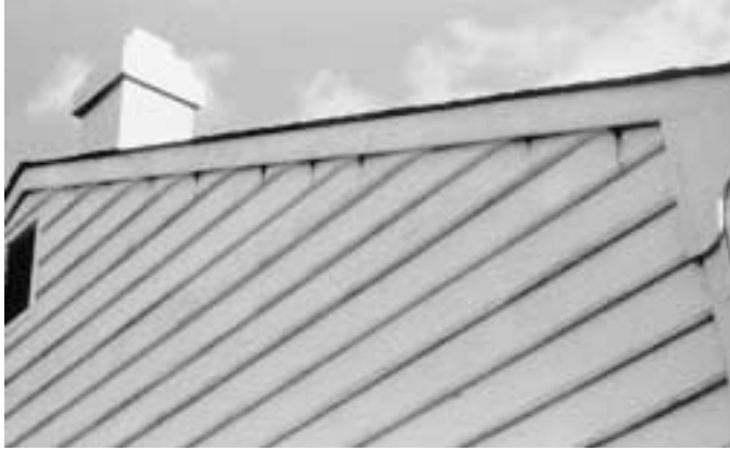
Figure 6.20. Carpenter bee damage.
