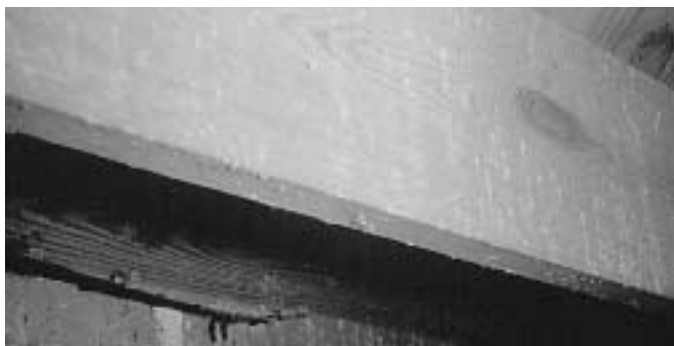
Figure 6.2. Anobiid beetle damage in pine floor joist—note frass being pushed out of old exit holes (USDA Forest Service).
