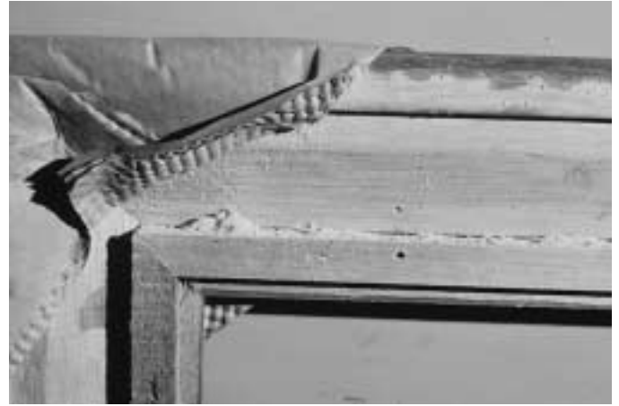
Figure 6.11. Lyctid beetle damage in framing around mirror (USDA Forest Service).
