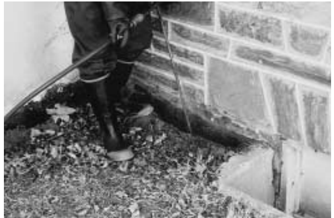
Figure 4.7. A typical basement treatment will also include trenching and rodding the outside perimeter of the foundation.
