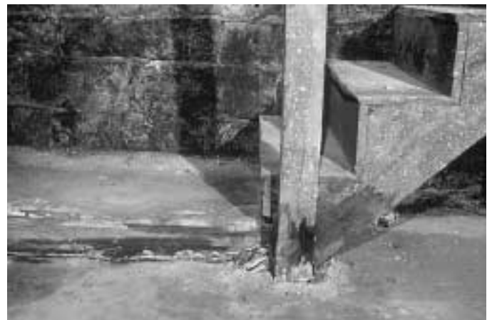
Figure 3.14. To prevent termite infestations, do not allow wood form boards to be embedded in concrete as shown in this basement.
