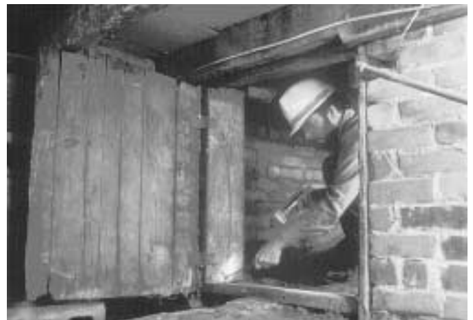
Figure 3.9. Inspection of crawl space for termite infestations (he should also be wearing gloves).
