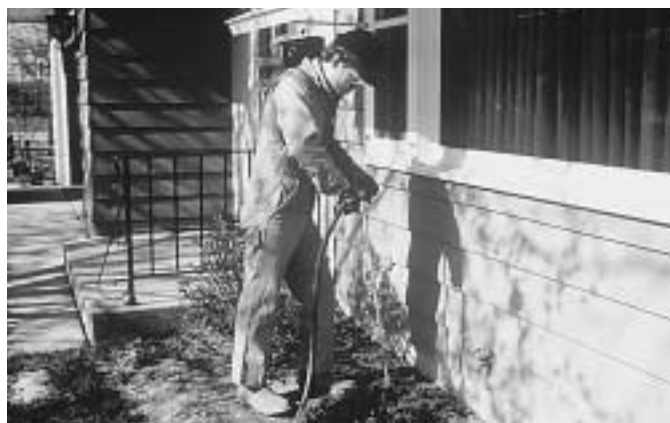
Figure 3.3. Pest management professional applying termiticide to the soil by long rodding the exterior of a house.
